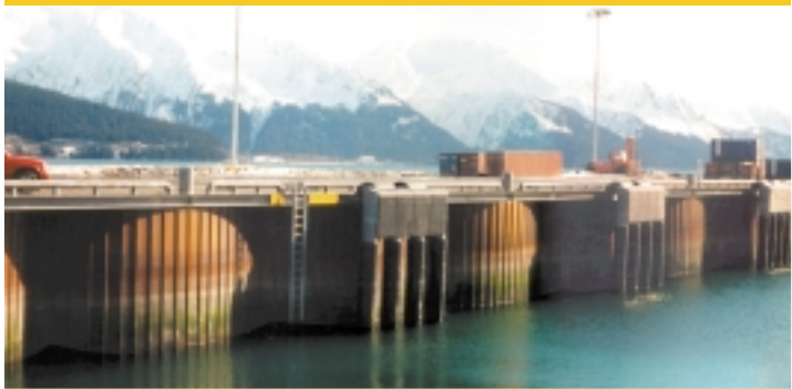
▶ Open Cell Dock, Seward, Alaska
