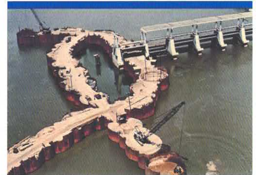
Going from the Stage 1 cellular cofferdam to the Stage 2 cofferdam in order to complete a Lock & Dam.
