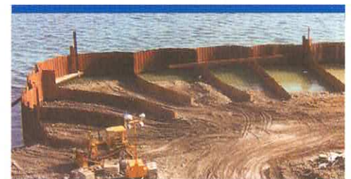
A USCG open cell dock with 70 foot face sheets under construction in Unalaska, AK.
