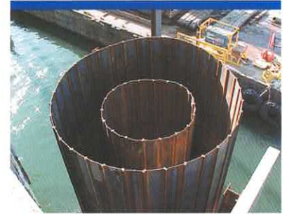
Reinforced pier protection cell under construction on the Mystic River in East Boston, MA.
