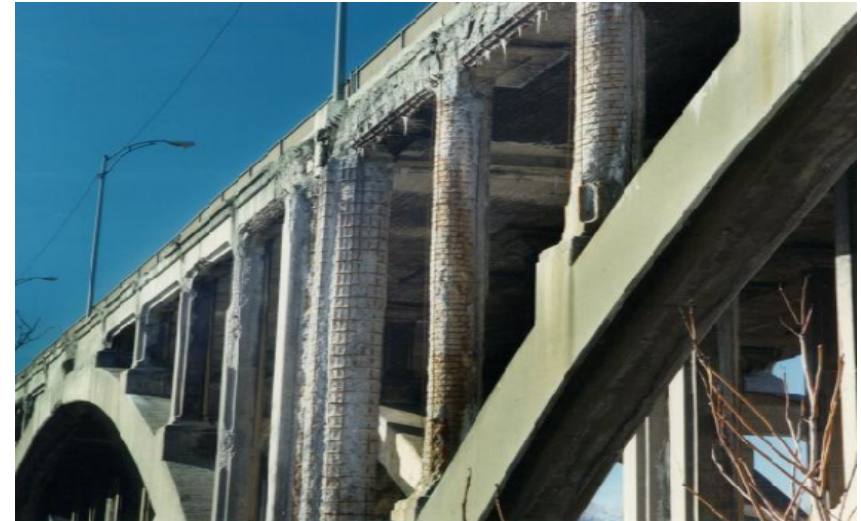
Example of concrete structure exposed to elements; deterioration starts from within
